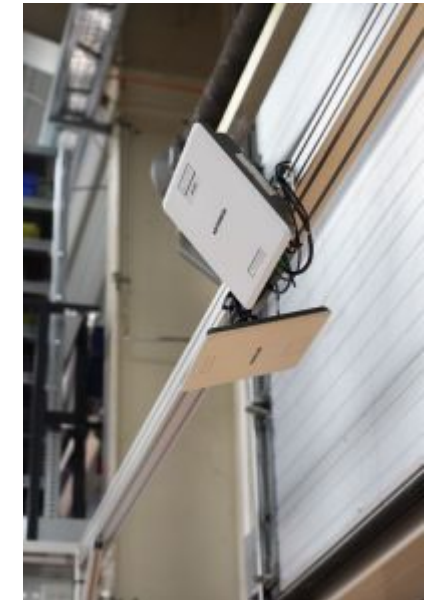
KATHREIN RRU 4500 Readers were installed directly above the loading gate.
